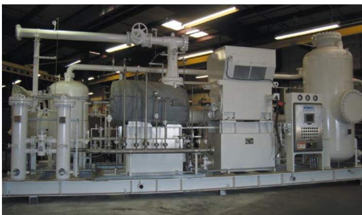
Figure 5. Typical oil injected screw compressor package for refinery platformer hydrogen service.
