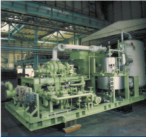
Figure 7. Typical oil injected screw compressor package for natural gas used fuel gas booster to gas turbine.
