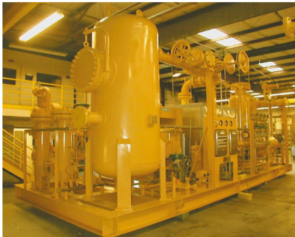
Figure 6. Typical oil injected screw compressor package for refinery offgas used fuel gas booster to gas turbine.
