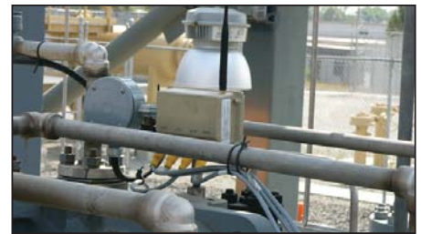
Figure 2: Wireless condition monitoring provides early warning of booster packages
