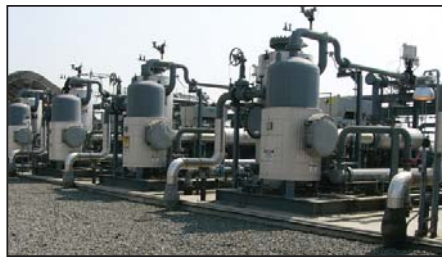
Figure 1: Five Kobelco screw compressors provide fuel gas boosting in Mountainview
