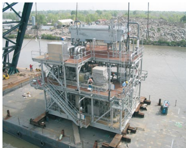
Figure 5. Oil free screw gas compressor for vapour recovery service on offshore platform.
